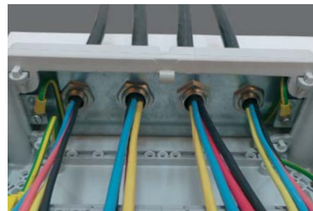
Cable entry for armoured cables via metal glands
