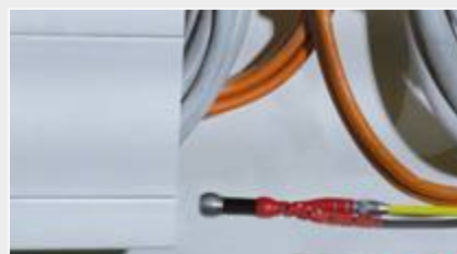
Shafts and underfloor ducting
