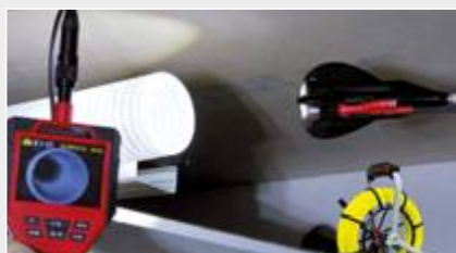
Ventilation inspection and servicing
