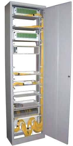
Only Front Access type (Depth 300mm) 1,000-port Termination Rack SC connector , Splice Tray
