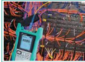
Fiber optic power test
