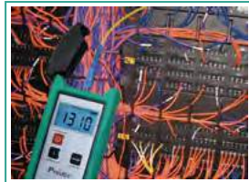
Fiber optic power test
