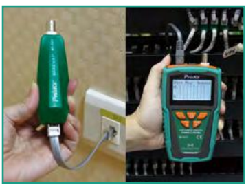
Verify LAN/ Telephone /Coaxial cable condition
