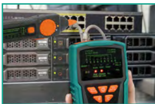
PoE switches & wire tracing
