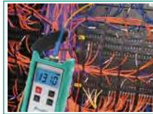
Fiber optic power test
