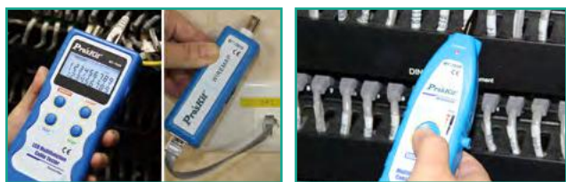
PoE switches & wire tracing
